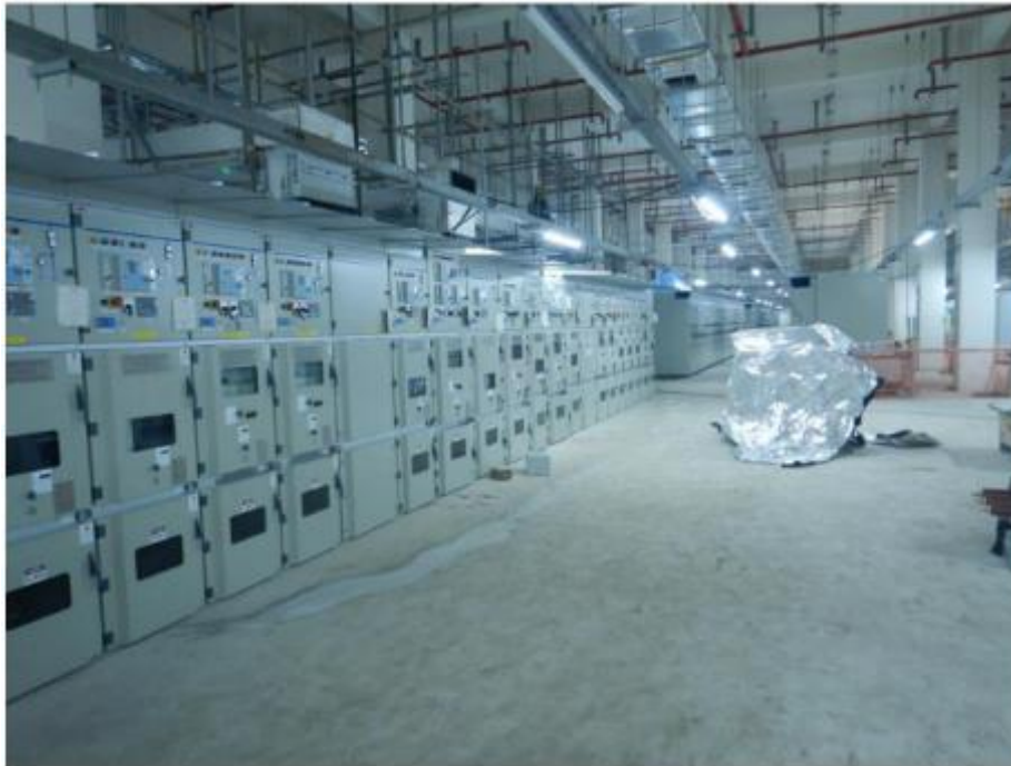
Gambar 5. Kondisi operasional Utilities Substation di PT Kilang Pertamina Balikpapan
